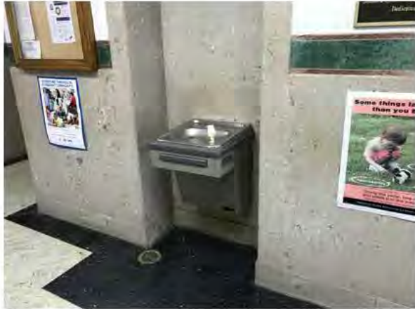
Lobby wall hung electric water cooler
