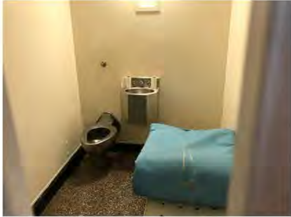
Jail Cell Men's /Women's water closet/lav sink
