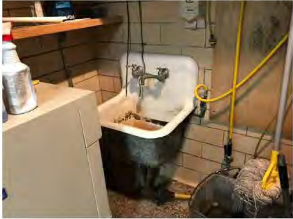
Original Service Mop Sink (Typical)
